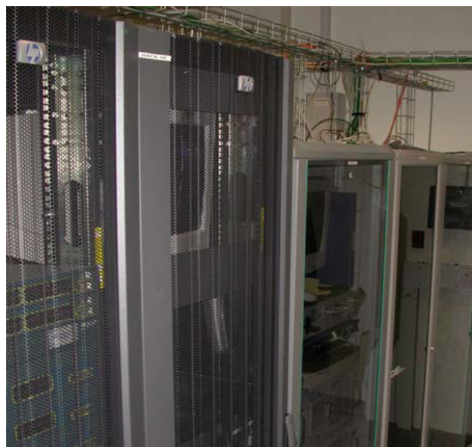
Server cabinets in one of the communication rooms
