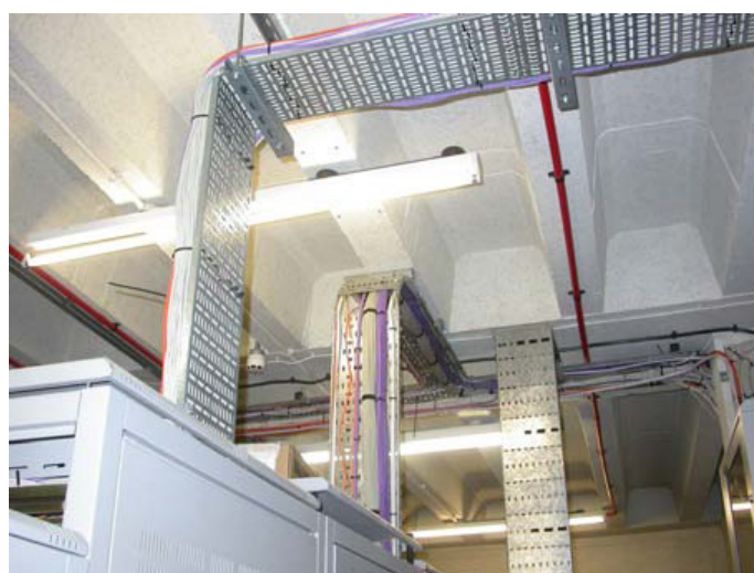
Structured cabling dropping into the communications room
